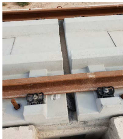
Figure 3: Groove in the concrete floating slab.
