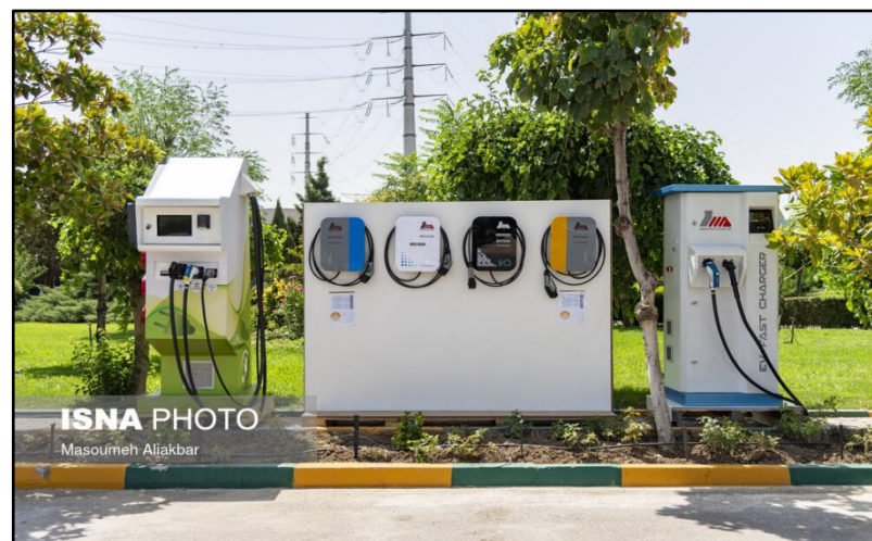
Figure 4. A PV-based charging station for EVs in Tehran, Iran [Photo by ISNA News Agency] [41].
