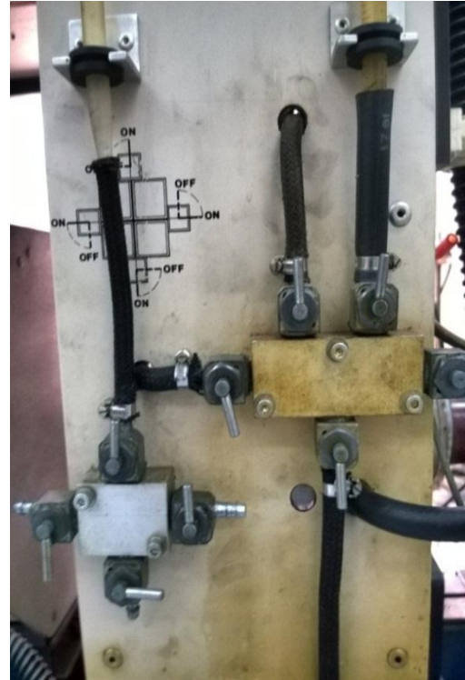
Figure 36. Fuel supply valves
