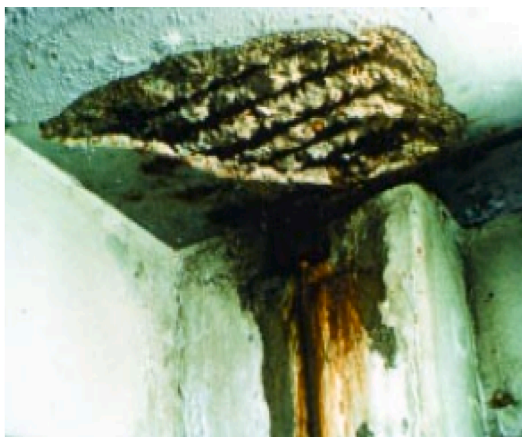
(a) Corrosion of reinforcing steel
