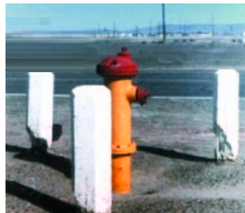
(b) Concrete posts suffered from a sulfate attack
