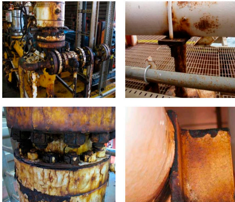
Figure 2. Example of corrosion effect on bolts, valves, flanges, piping, and pipe support [7].
