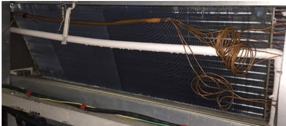
Fig. 6. External frost formed on the evaporator double pipe.
