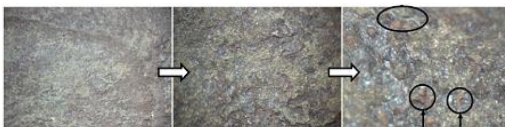
Figure 16. Zoomed-in views of the heavily eroded location (magnification increases from left to right)
