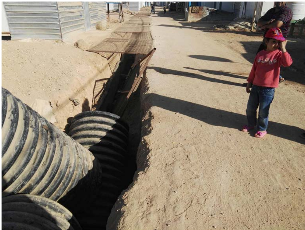
Figure 32: Unfinished infrastructure works (By: Suzan Manasrah, Nov. 2017).
