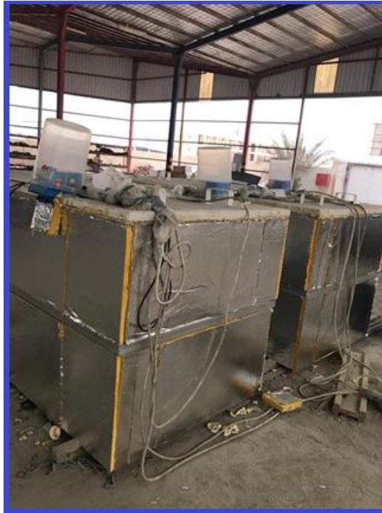
Figure 35: Steel Tanks Insulated with 2.5 cm Rockwool Sheets.
