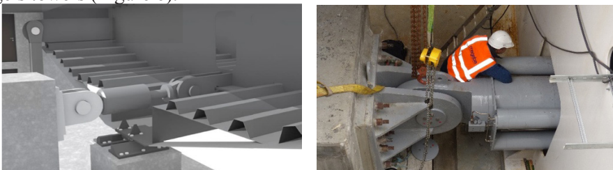
Figure 6: An STU at each tower of the Hålogaland Bridge controls superstructure movements – design representation (left) and during installation (right)
