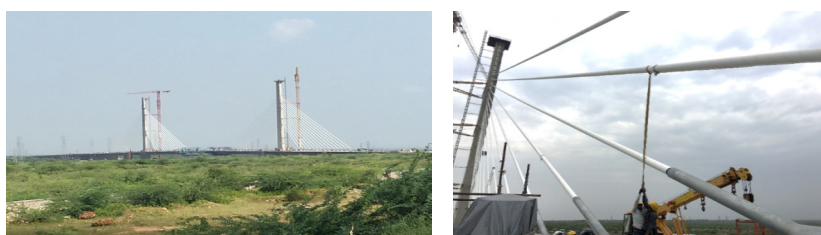
Figure 9: Construction of Kota Chambal Bridge (left), with monitoring of many variables including stay cable vibrations (the picture on the right shows forced vibration of a stay cable with an accelerometer)
