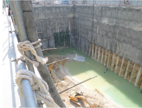
Figure 4: Water ingress inside the station due to karstic feature
