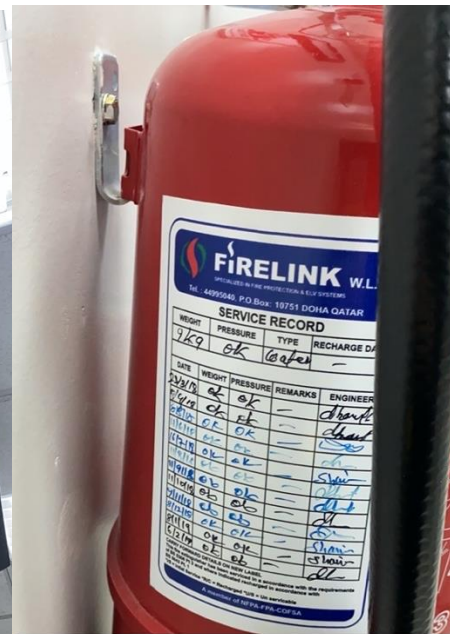
The water fire extinguisher is inspected
