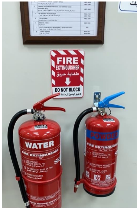
Appropriate fire extinguishers are available
