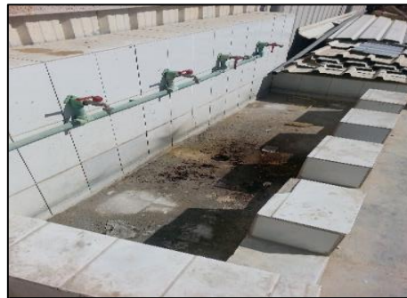
Sewer waste water at Shahania Animal complex
