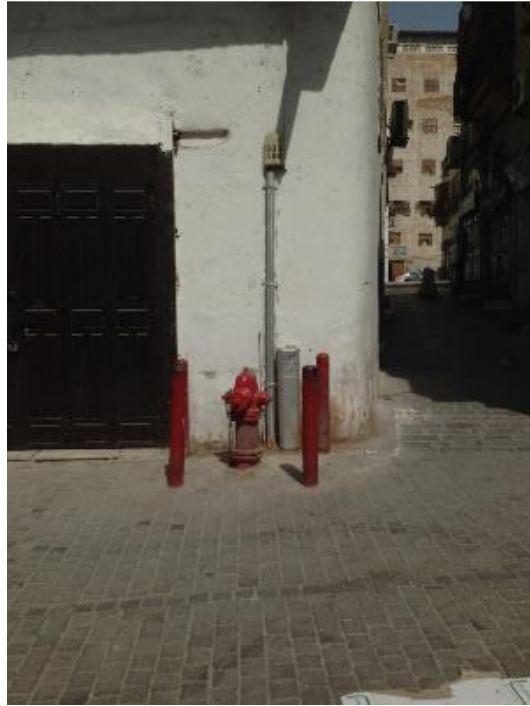
Figure 4-31. A Street Fire Pump (Source: Author)
