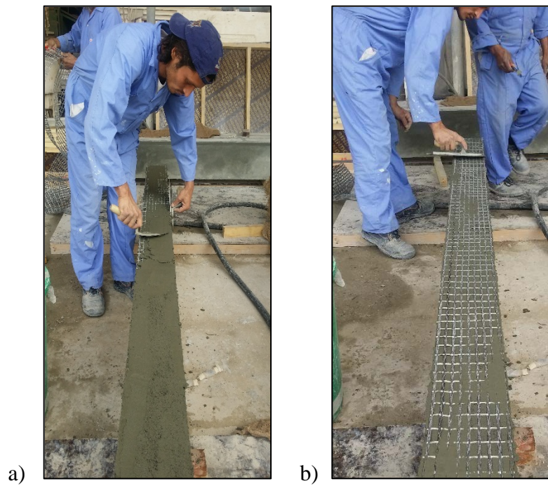
Figure 23: a) Laying the second layer of mortar and b) Textile over the second mortar layer
