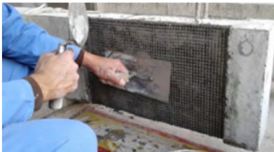
c) Installation and full impregnation of first layer of fabric (full configuration).
