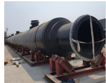
HDPE pipework transition
