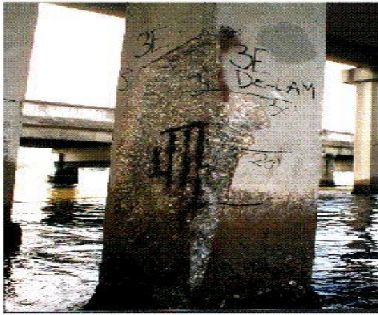
(a) RC deterioration
