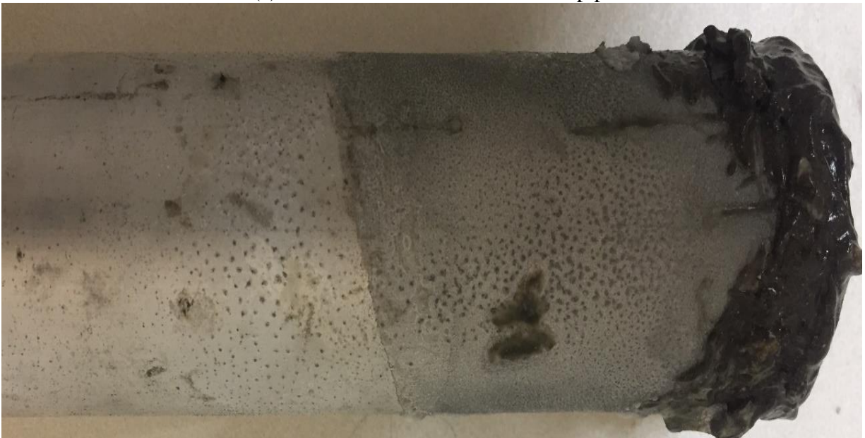
(b): Corrosion in non – joined aluminum pipe
