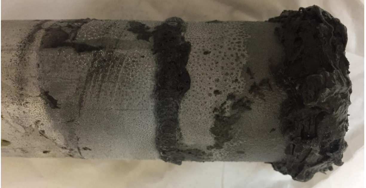
(a): Corrosion in welded aluminum pipe
