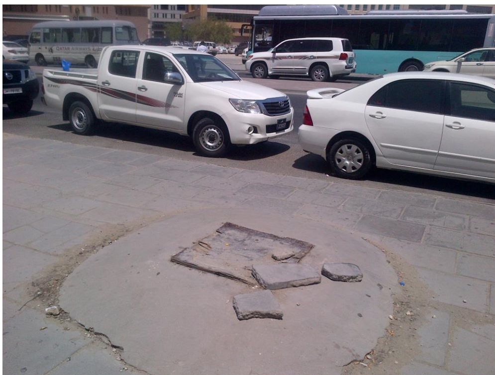
Figure 18. Manhole related complaint
