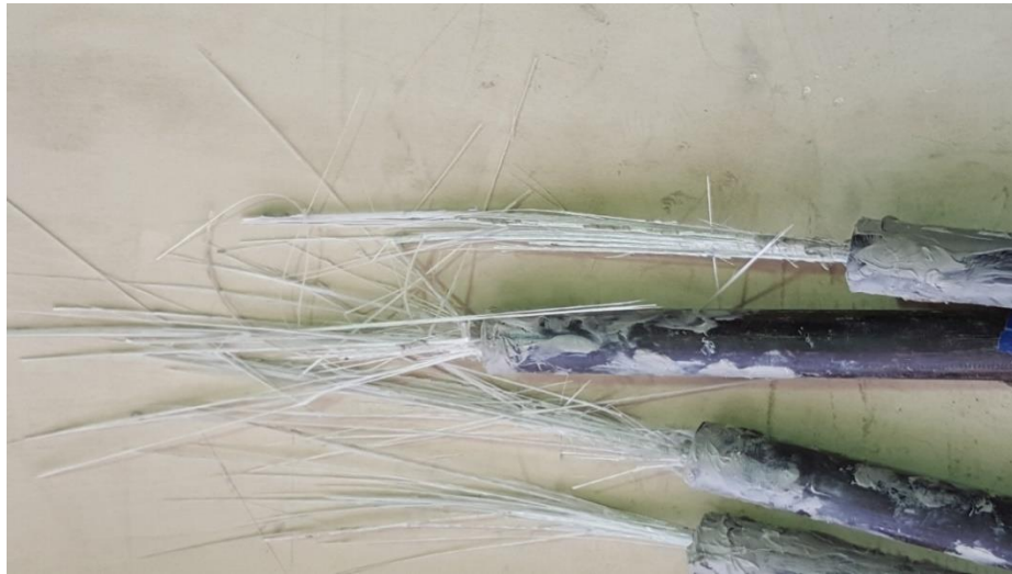
Figure 21. GFRP Reinforcing Bars after Failure
