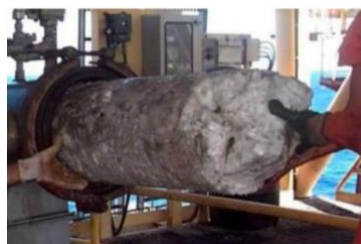
Figure 1. Remediation of a hydrate plug in natural gas transportation pipeline [14].
