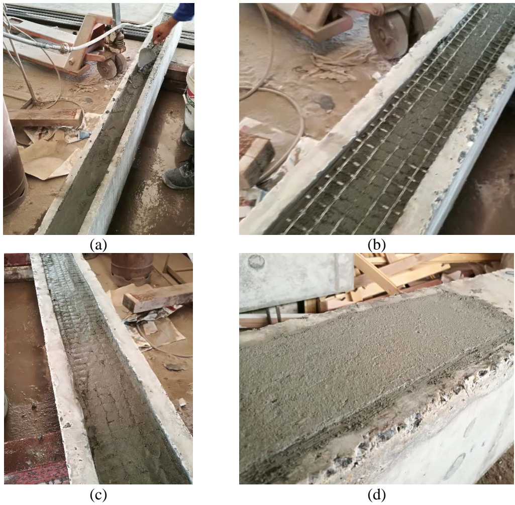
Figure 9 NSE-FRCM application: a) applying the first layer of mortar, b) placing the first layer of fabric, c) impregnation of fabric, and d) finished surface for NSE beams
