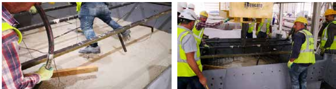
Figure 13: Site cast concrete pouring on top of Robotically Adaptive Molds (RAM) creating the shell cassette inner interior substructure.
