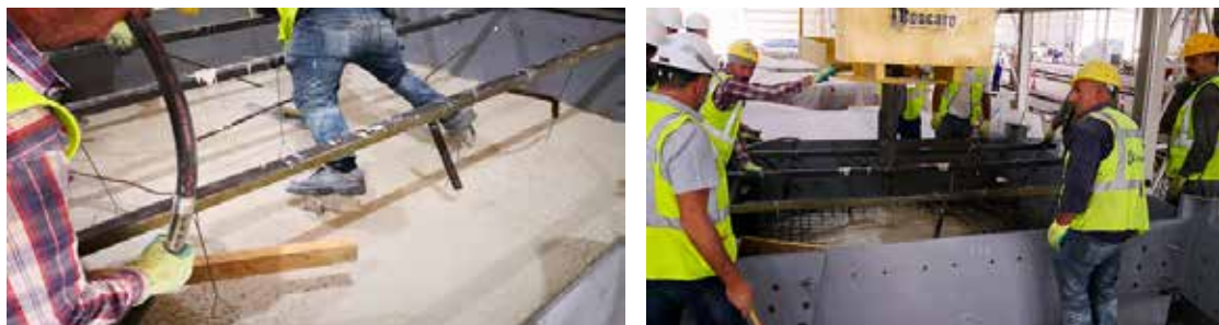
Figure 13: Site cast concrete pouring on top of Robotically Adaptive Molds (RAM) creating the shell cassette inner interior substructure.
