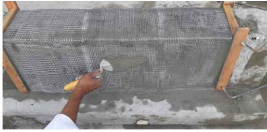
(a) Bonding the first layer of the steel fabrics and impregnating with the matrix
