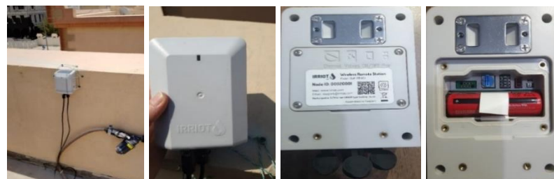
Figure 52. Remote wireless valve control station of IRRIOT system.
