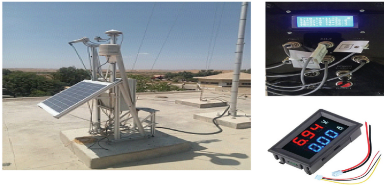
Figure 2. Weather station, data logger and VOLTAM meter.
