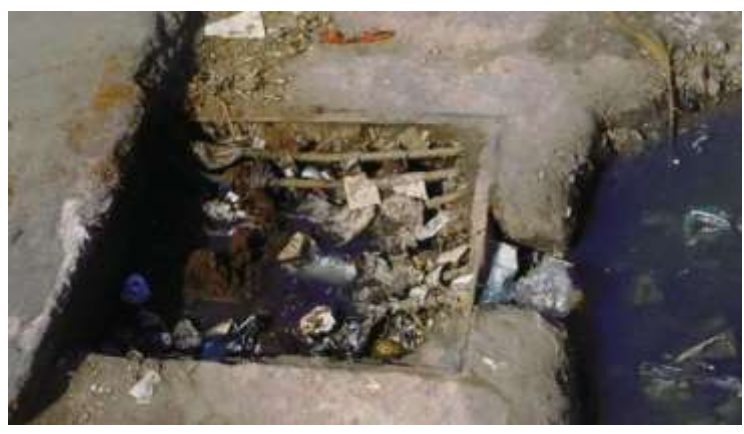
Figure 81: Clogged entrance to storm water drain. Source-Chennai pollution board.
