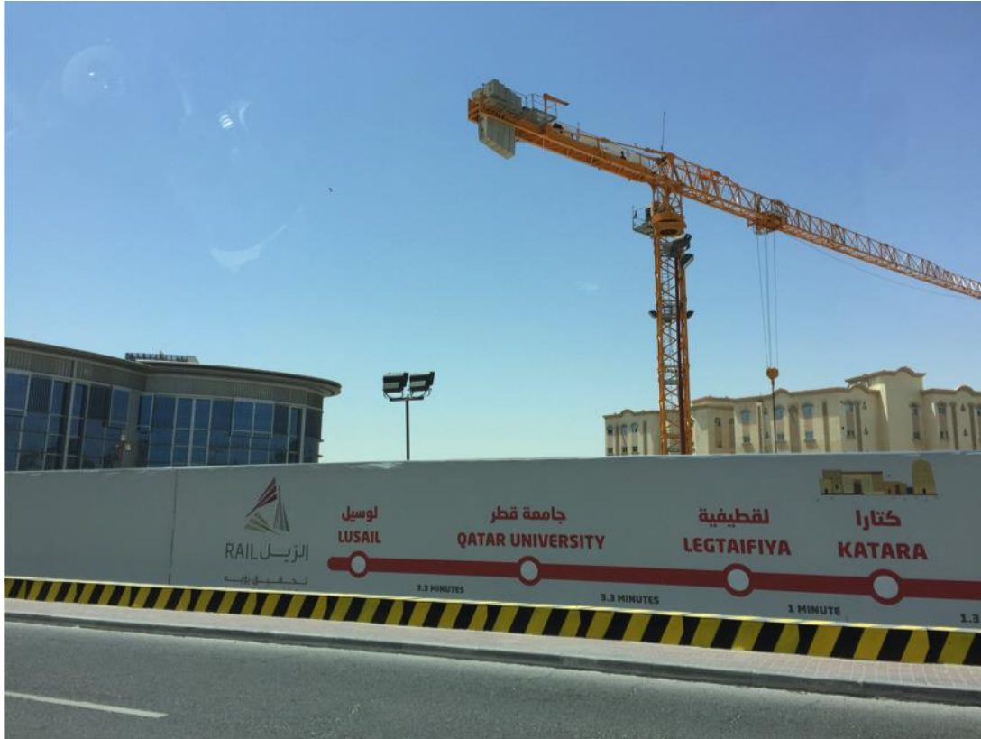
Figure 36: Najma Metro Station Construction Site, Photo taken in April 2016. Source: Author
